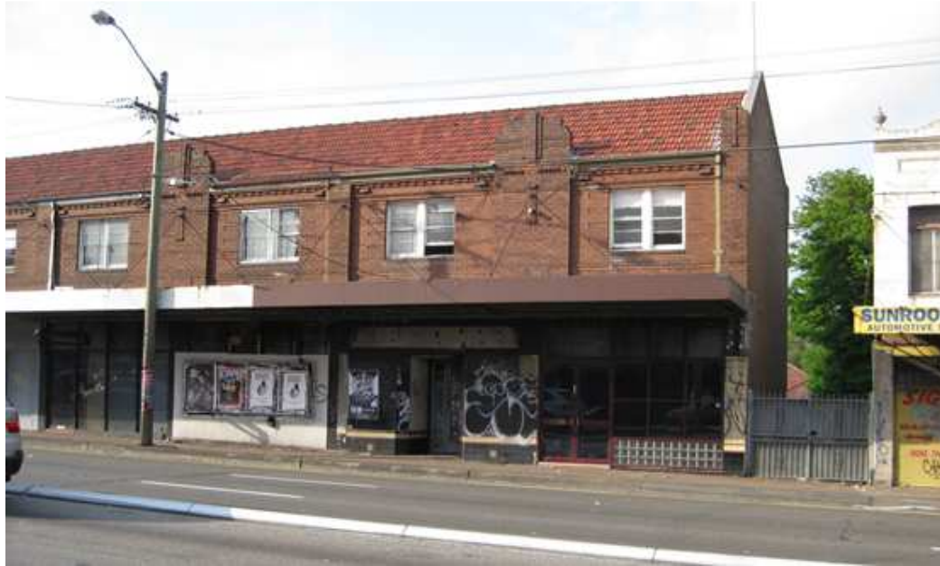
Figure 3 – Derelict properties on Parramatta Rd.
